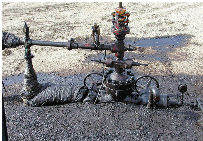
Above: An example of the kind of heavily leaking wellhead that oil companies sometimes have to deal with.
