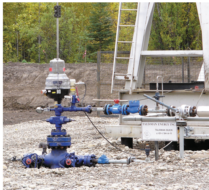
Right: A clean site using Titan spill containment technology, which features packing failure blowout protection with high-level fluid shutdown capabilities for heavy leaks.
